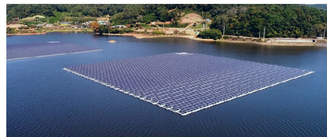
Floating Photovoltaic System
