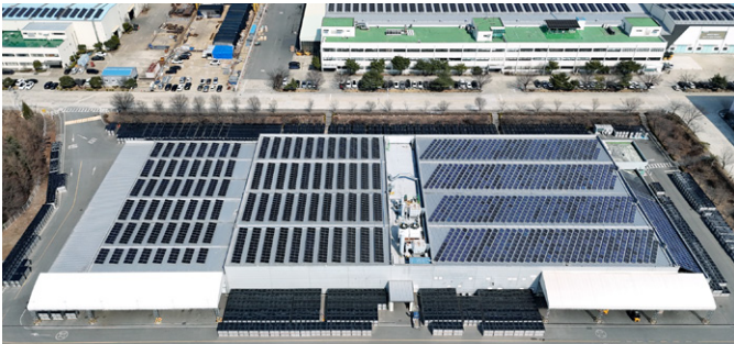
Solar Power System of Eumseong Module Plant 3
