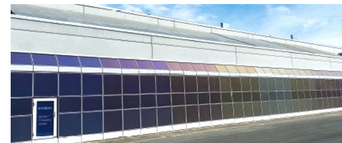
Building-integrated Photovoltaic System (Eumseong Plant)
